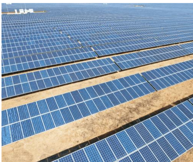
Mahindra Renewables solar power installation, Madhya Pradesh
